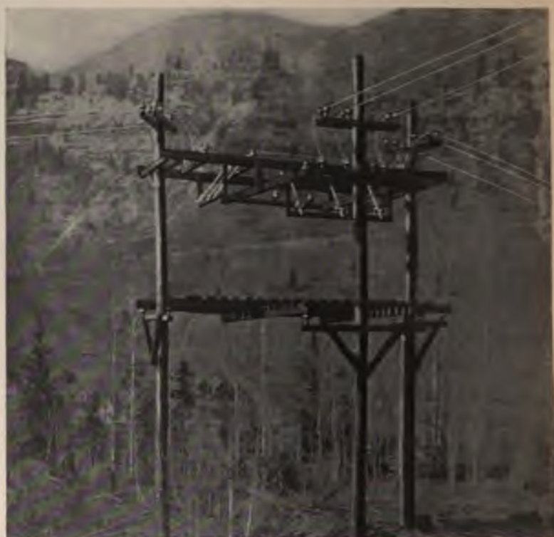
FIG. 2.— AN OPEN-AIR SWITCHING JUNCTION.
